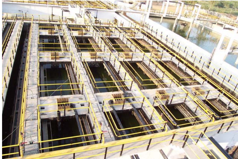
Fig. 4.5. Location of final distribution boxes on top of a UASB reactor.
